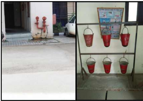
Fire Fighting Equipment
