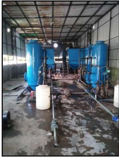
Sewage Treatment Plant
